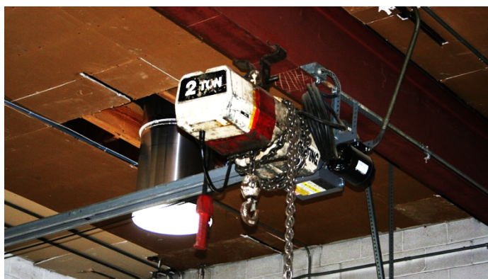
2 TON CRANE & 14.4' CEILING HEIGHT
